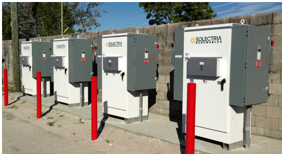
Figure 29: Central Inverters Example
